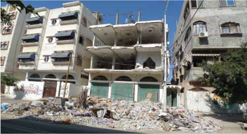
Damage caused by a 'roof-knock' strike and by the main strike that followed it, Beit Lahiya, north Gaza.
